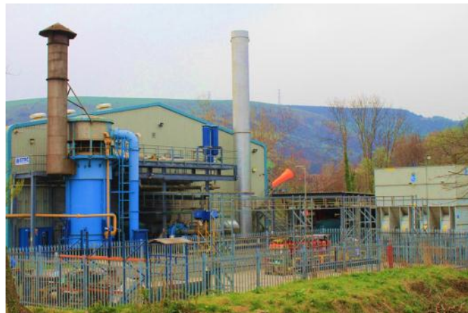
Figure 1: Cardiff University's GTRC facility, which shows the gas storage area in the foreground.
