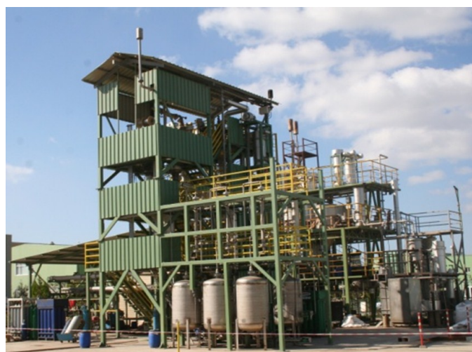
Figure 2: Pilot Scale Bubbling Fluidized Bed Gasifier.
