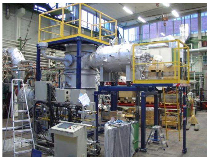
Figure 1: 500 kW High Temperature Air and Steam Gasification (HTAG) test facility.
