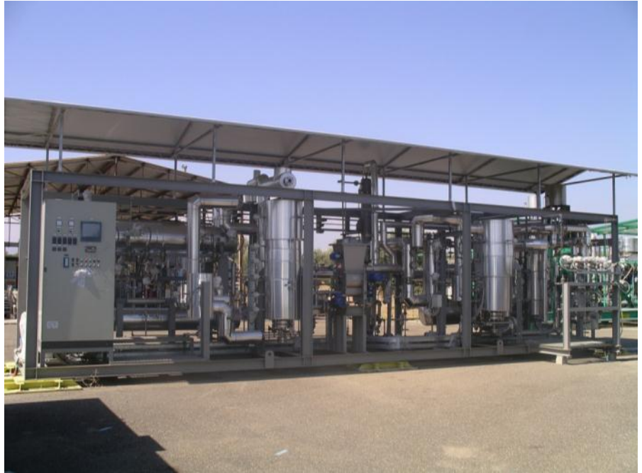
Figure 1: Hydrogen from waste. In this plant 5 kg/h of plastics can be gasified through a bubbling bed fluidized with mixtures of oxygen, water steam and air. The gas produced is then cleaned and catalytically upgraded into a hydrogen rich stream.
