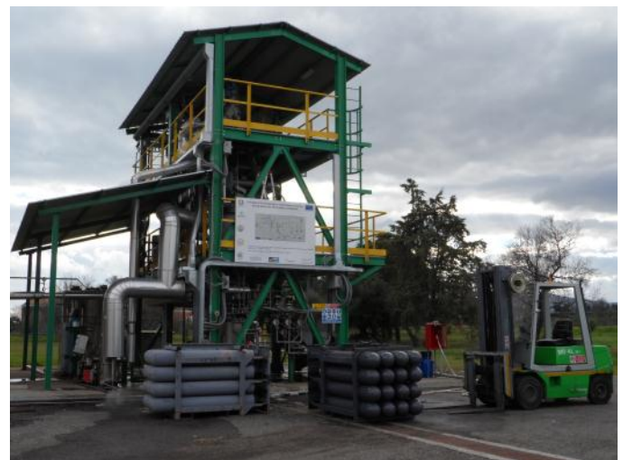
Figure 4: ENEA's facility for fixed bed gasification and gas cleaning (ground and first floor), and syngas upgrading (second floor).
