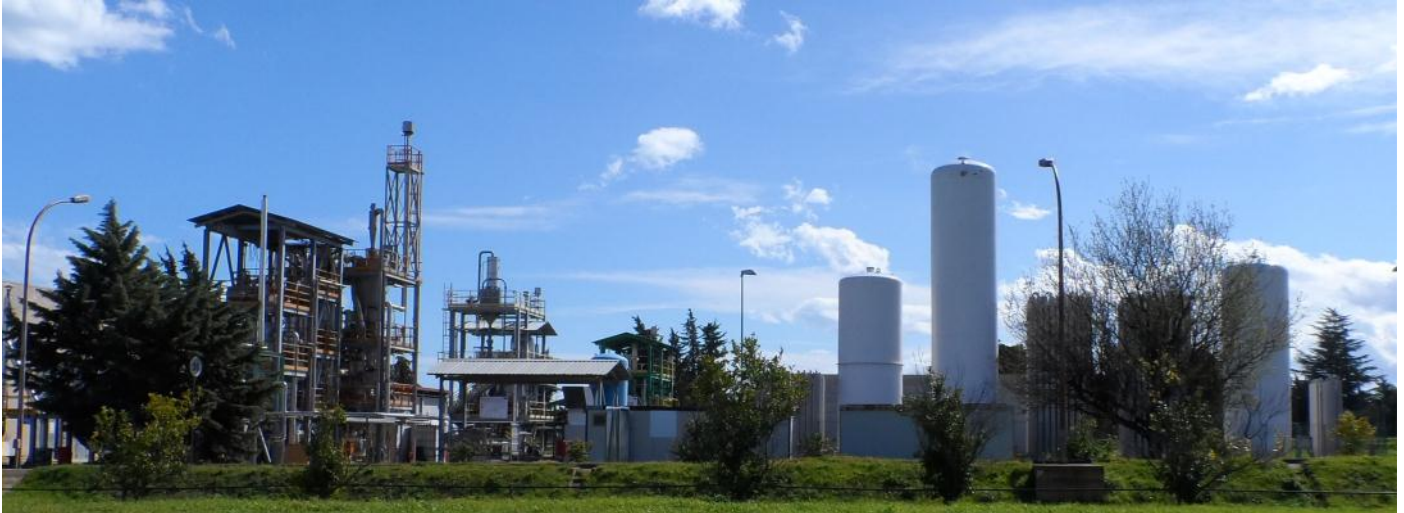
Figure 3: ENEA's Trisaia Research Centre – biomass gasification plants. Scales from 10-1000 kW th are available; fixed bed (down and updraft) and fluidized bed (bubbling and recirculating) technologies are tested.
