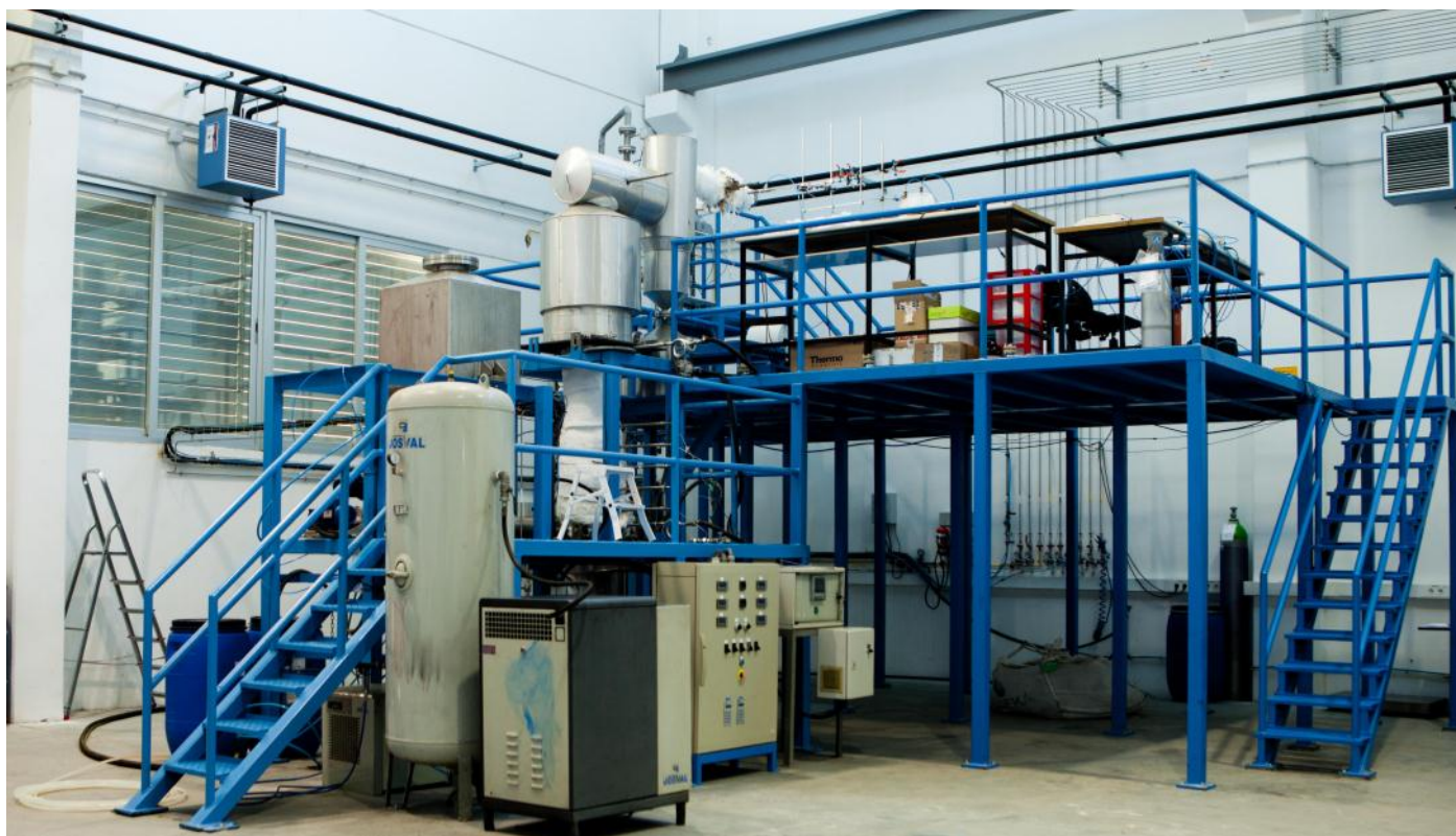
Figure 1: Biomass pilot scale fluidized bed plant at GPT-UNIZAR laboratories.
